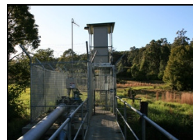
Porters Creek Pump Station (source: Wyong Shire Council)
