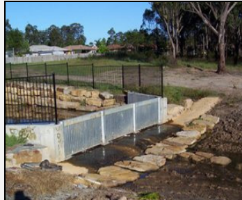
Outlet from the GPT
